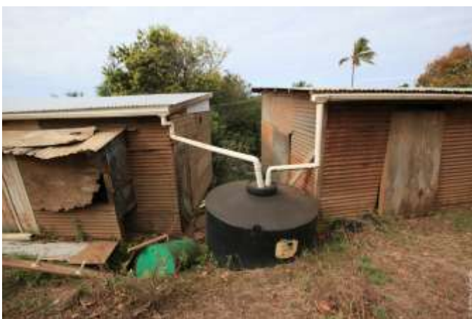
Figure 16. Rainwater harvesting (as drinking water)
