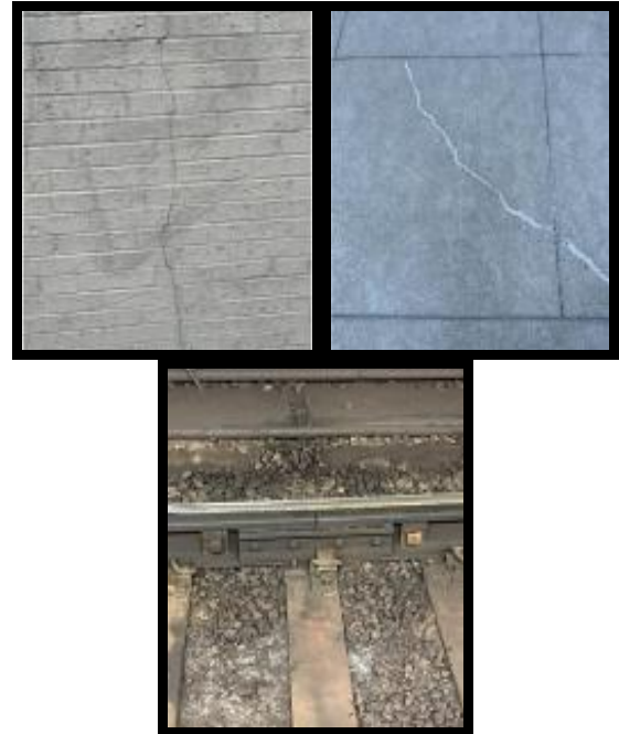
Figure 12: Pictures observed in buildings, walkways, and railways as an application of Fracture in Brittle (brick and concrete) and Ductile (steel and iron).
