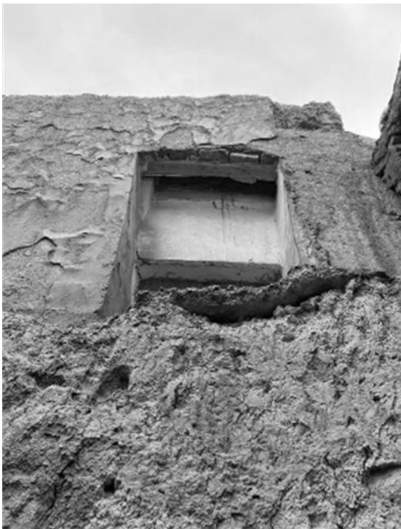
Figure 3. Damage to the roof has caused the complete destruction of the windcatcher in Herat's old city. (Source: K. A. AHMADI)
