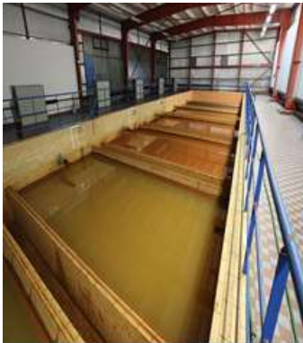
Fig. 2. Tanks with sand filters to remove sedimented iron (not working at that time)
