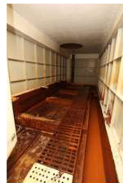
Fig. 1. Empty aeration tank for iron deposition
