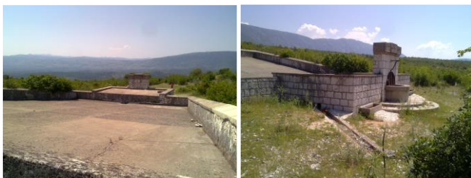
Figure 21. Large water cistern ('state catrnja') in the Osanici village near Stolac (built in 1934)
