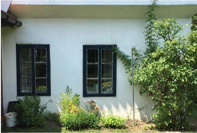
Figure 10. The Gradascevic family house in Gradacac. Windows in the ground floor residential unit
