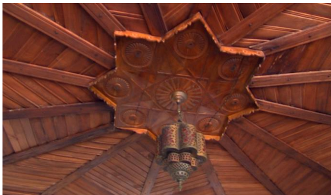
Figure 11. The Biscevic family house in Mostar. Wooden ceiling ('shishe') in the hall on the first floor of the house ('visit-room') Source: https://www.youtube.com/watch?v=ckmKTf4hlu4&t=87s , Accessed: May 28, 2023.
