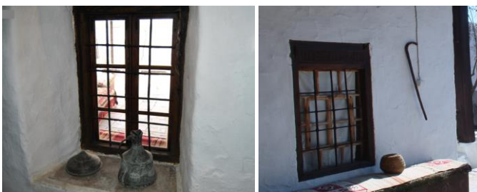
Figure 12. The Kajtaz family house in Mostar. Windows on the ground floor of the house
