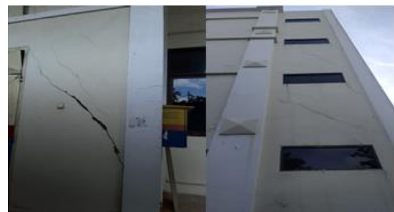
Fig. 3. Damage to the Bappeda Kukar building
