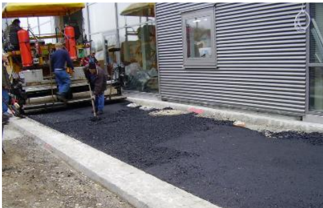
Figure 11: Manual laying of the asphalt with PmB bitumen on a construction site belonging to the author [K. Hrapović, 2006]
