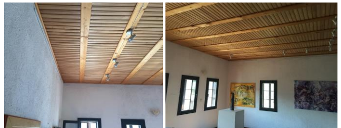
Figure 18. Krslak's house 01. Ceiling at floor level - towards the attic
