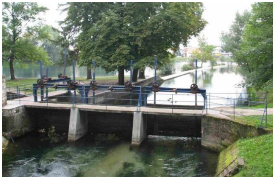
Figure 20. Hydroelectric power plants on Jarak (“Mala HPP Bihac” or “HPP Jarak” or “HPP Kanal Una”)
