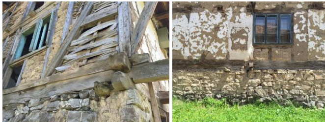
Figure 20. The Colak family house in the Brnjic village near Kakanj. Construction and materialization, walls
