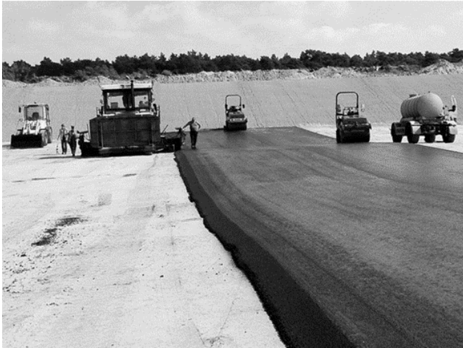
Fig. 27. "Hot to hot" asphalt base courses on geological barrier with inclined seam flank [22]
