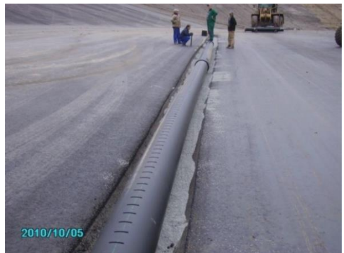
Fig. 7. Pipe support a landfill with PE-HD seepage pipe [5]
