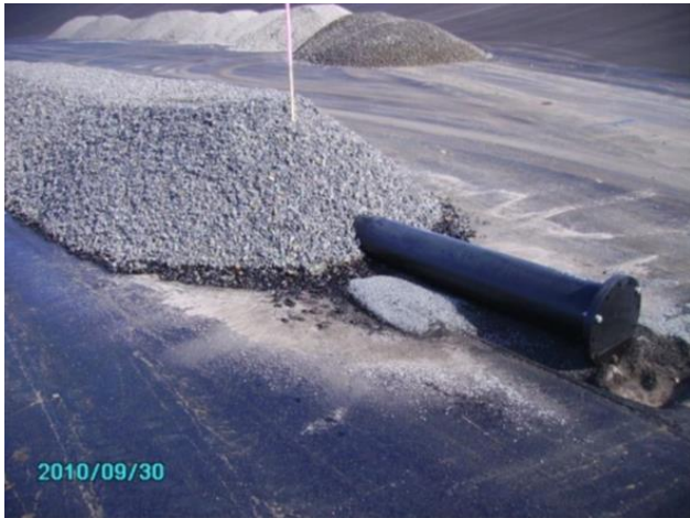
Fig. 9. Pipe support a landfill with PE-HD seepage pipe and drainage layer of gravel 16/32 mm [5]
