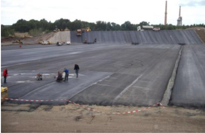
Fig. 17. Asphalt paving work at the Wetro "Puschwitzer Feld" industrial waste disposal site of P-D Industriegesellschaft mbH, Puschwitz, Germany [5]
