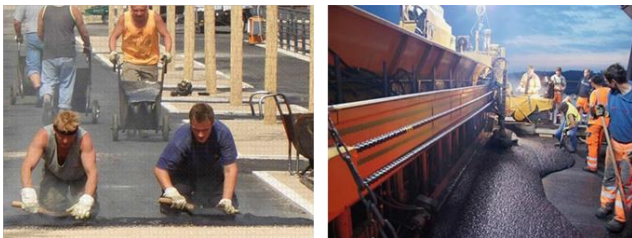
Figure 6. a) Manual laying of mastic asphalt [1]; b) Paving mastic asphalt by machine [1]
