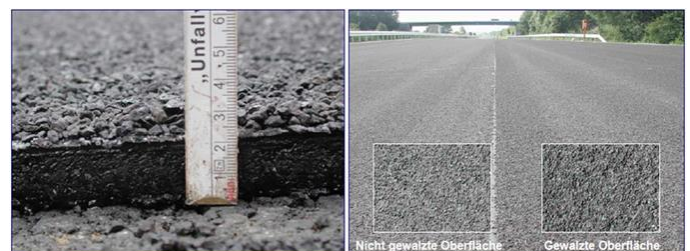
Figure 9. a) Paving MA on a German highway, 2cm thick when installed [1]; b) Left: unrolled highway surface, right: rolled highway surface [1]
