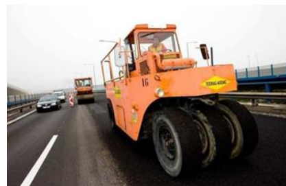
Figure 8b. Rolling in the hard chippings of mastic asphalt using rubber roller and smooth wheel roller [1]
