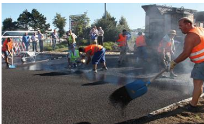
Figure 7a. Asphalting of the roundabout in Hartberg in Styria on the B50 in 2011 (Styria) [1, 6]
