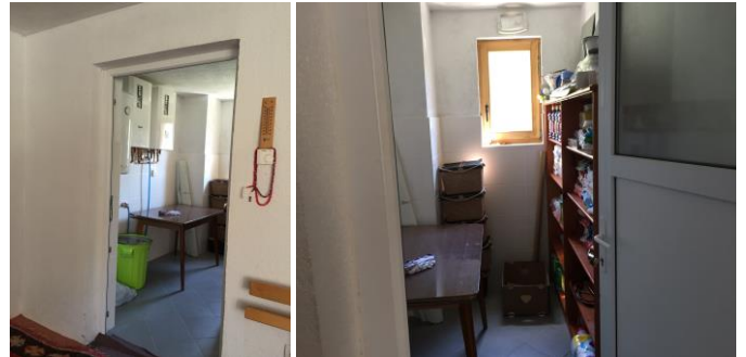
Left: View into the room for the preparation of central heating from the tavern (basement)
