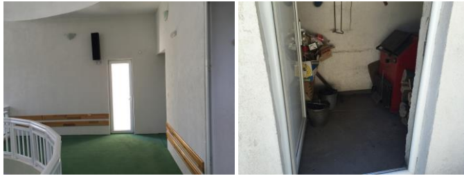
Left: Exit to the minaret from the mahfil Right: Boiler room for central heating Figure 3. Mosque in Japalaci near Tarcin Source: Author (July 14, 2017)
