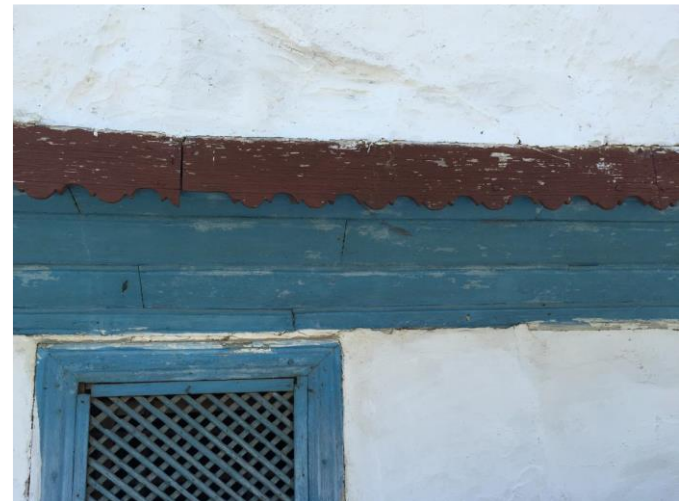
Figure 14. Decorative cornice made of profiled boards, a border that emphasizes the transition from the ground floor to the first floor
