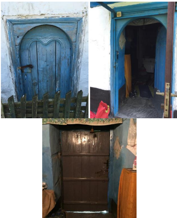
Left: The door at the entrance to the ground floor directly from the street In the middle and on the right: The door at the entrance from the courtyard to the hayat (ground floor)
