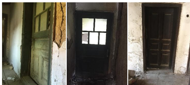
Figure 26. Door annex-hallway of the residential floor on the first floor (left and middle) and door on the loggia (right)
