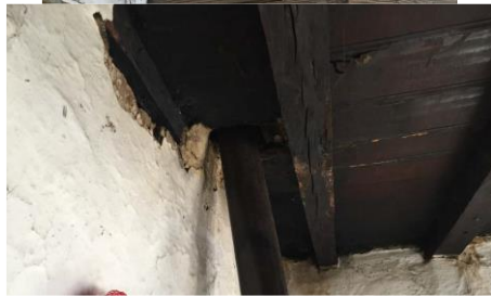
Figure 7. The floor is made of thick, roughly worked boards. Fire protection of flue penetration from the ground floor into the attic (left) and floor-attic construction in the sofa area (divanhana)
