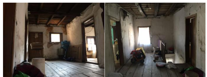
Figure 5. Upstairs divanhana space oriented to the courtyard and the Sana river (left) and street divanhana space oriented (right)
