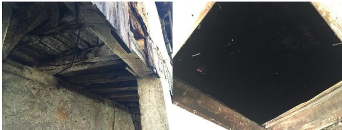
Figure 21. Interfloor structure in the part of “vodnica” (left) and the roof structure is of the type “horns with a crucifix” (right)
