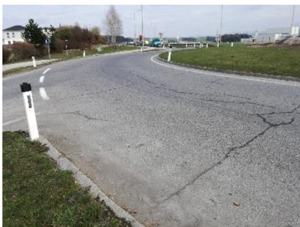
Fig. 8. Damage in the carriageway of a roundabout designed as a semi-rigid wearing course [8]
