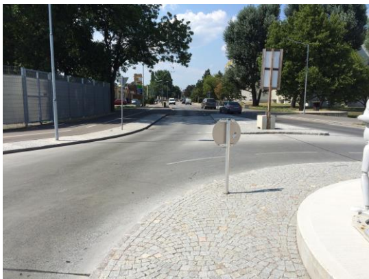
Fig. 10. Very good condition of the semi-rigid pavement of a roundabout years after installation [8]
