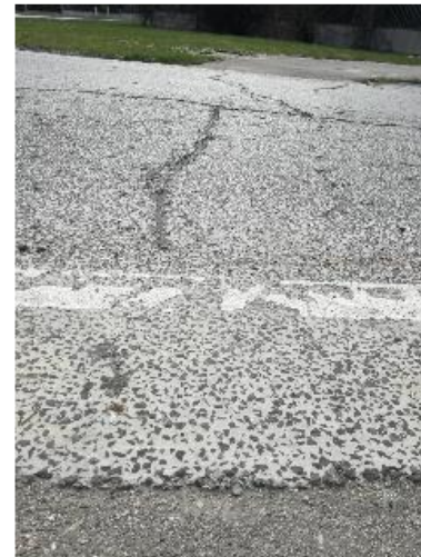
Fig. 9. Damage in the carriageway of a roundabout, designed as a semi-rigid wearing course [8]
