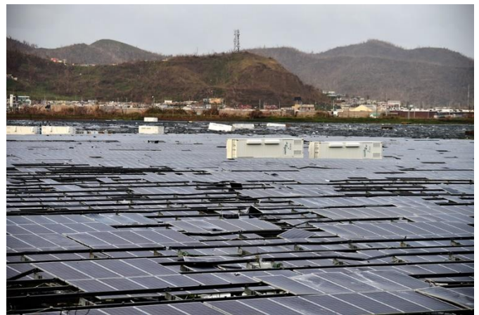
Fig. 4. solar panel facility in Humacao, eastern Puerto Rico was wrecked (BloombergNEF, 2017).
